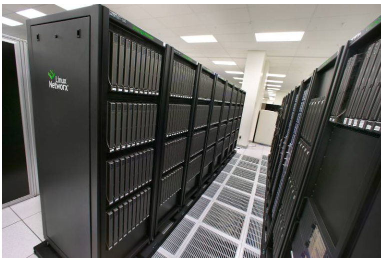
Figure 11. Jacquard is a 722-processor Linux Network Evolocivity cluster system with a theoretical peak performance of 2.8 teraflop/s.
