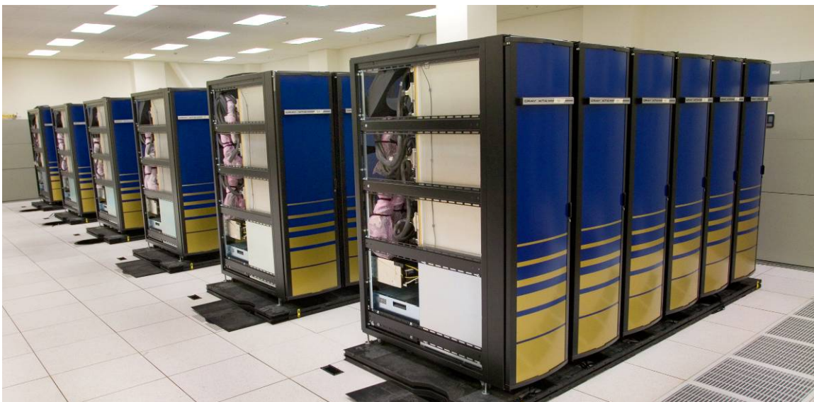
Figure 14. The first 36 cabinets of NERSC’s Cray XT4 supercomputer, which, when complete, will deliver sustained performance of at least 16 teraflop/s.
