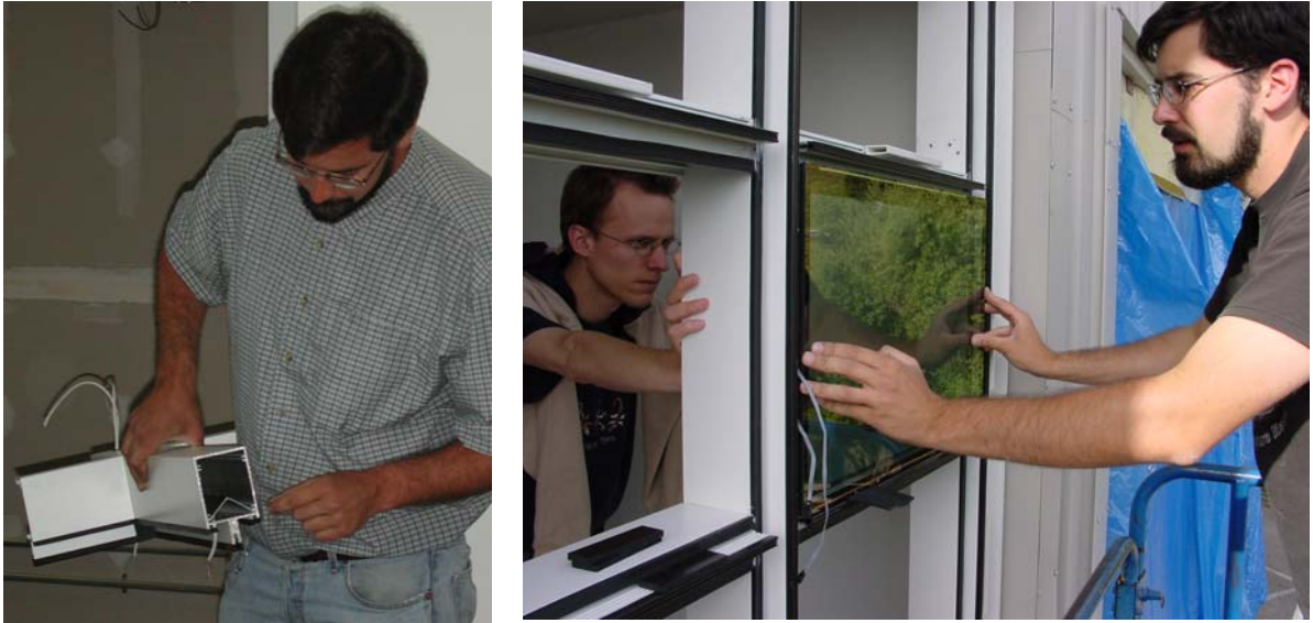
Figure 11. V-channel used to thread cabling through the vertical framing members (left). LBNL installation of EC windows using an exterior-mounted curtainwall system (right).
