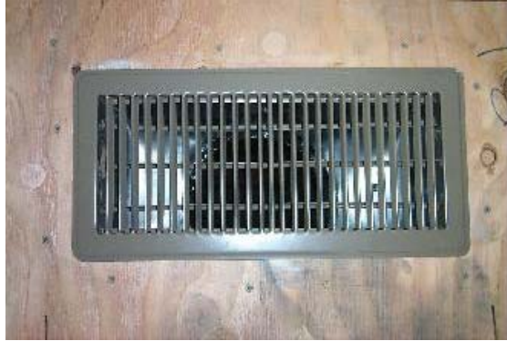
Figure 5. Example supply grille of multi-branch duct system in LBNL laboratory
