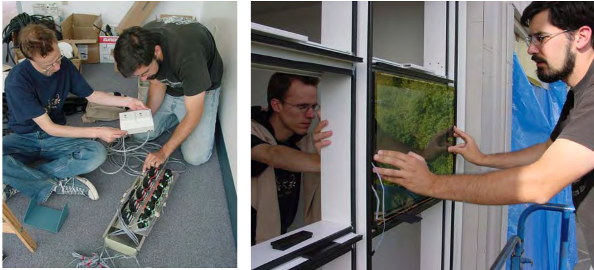
Figure 32. EC window controllers in the foreground (left) and installation of EC windows using an exterior-mounted curtainwall system (right).
