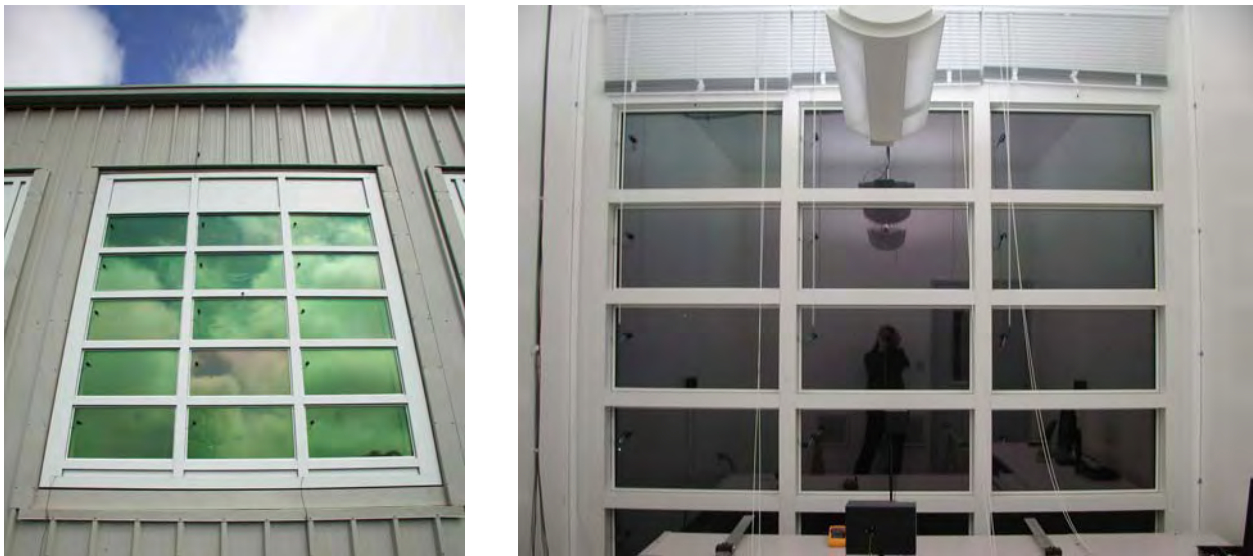
Figure 10. Exterior view of the EC windows on September 10, 2003 (left) and interior view of EC windows on July 5, 2005 (right).
