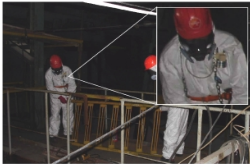
Fig 1: Personal air sampling by individual impactor during work area preparation, room G 635/3, mark +33
