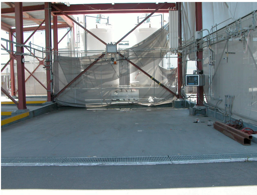
Figure 3-8. Area 514-1 Container Storage and Treatment Unit
