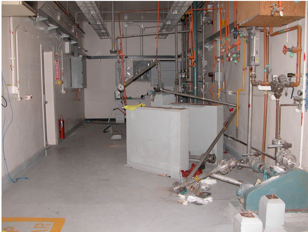
Figure 3-7. Wastewater Filtration Unit
