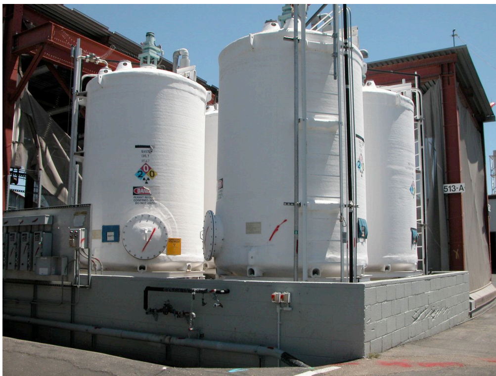
Figure 3-5. Quadruple Tank Unit
