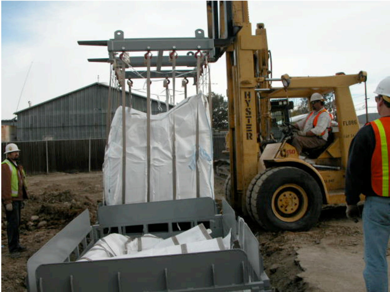
Figure 6-2. Lift liners Used for Management of Low-level Radioactive and Mixed Waste Concrete Rubble
