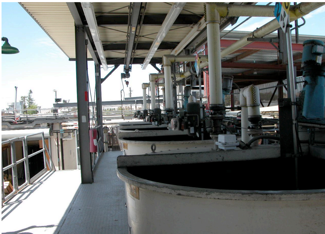
Figure 3-3. Wastewater Treatment Tank Farm
