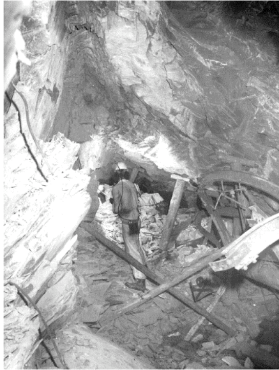
a) Unsymmetrical roof collapse and floor rubble due to a rock burst in a South Africa gold mine (courtesy of Dr. Ortlepp, 2003)
