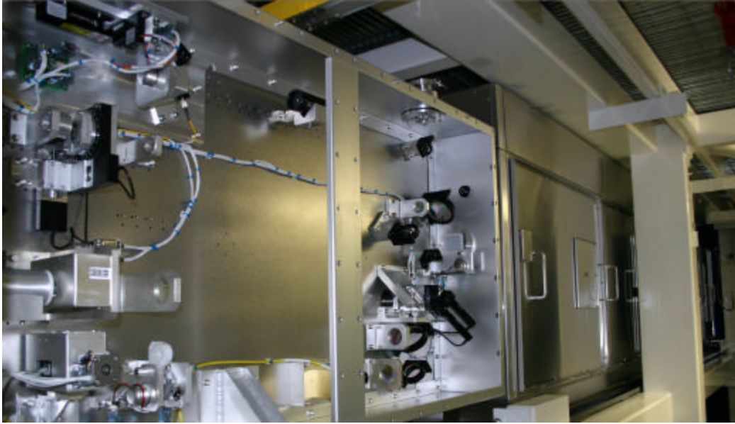
Figure 14. The ISP diagnostic side installed in NIF adjacent to an installed PAM
