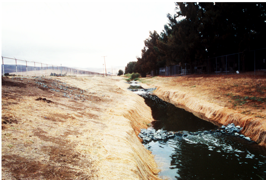
Figure 50. Photograph of 3G after dredging activity during initial precipitation of the year. Note erosion control blankets used for bank stabilization and rock weirs used for grade adjustment.
