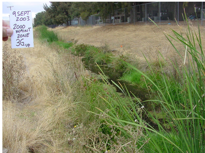
Figure 56. Photograph showing the lower end of Zone 3G (upstream view) three years after dredging with hydrophytes established and closing in on open water habitat.
