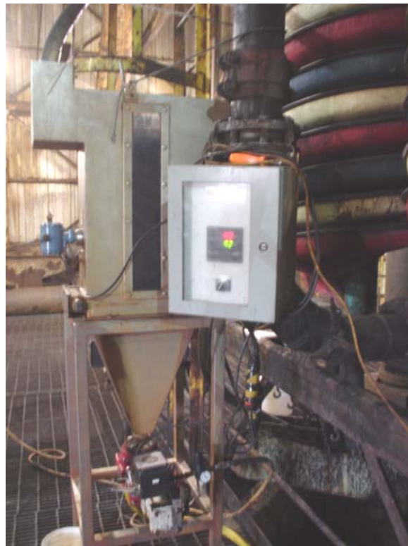
Figure 3.5. The 9x16 inch pilot-scale Crossflow circuit at Coal Plant B.
