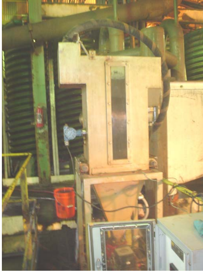
Figure 3.16. The 9x16-inch pilot-scale CrossFlow circuit at Coal Plant E.
