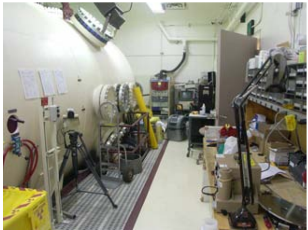
Figure 6.17 SNL ECF Large Walk-in Chamber, 1213A
