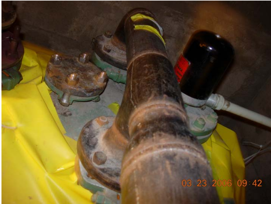
Figure 4. The 3-in. reactor drain tank vent line.
