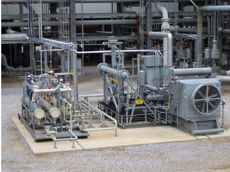
Figure 1. MTR's field demonstration membrane-based gas treating unit at BP Amoco's gas processing plant in Pascagoula, MS. The unit operated virtually continuously from December 2005-September 2006 with essentially constant conditioning performance.
