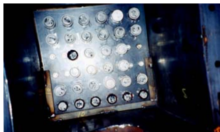
Photo No. 10. Rotatable Plenum Diffuser Plate - Closed
