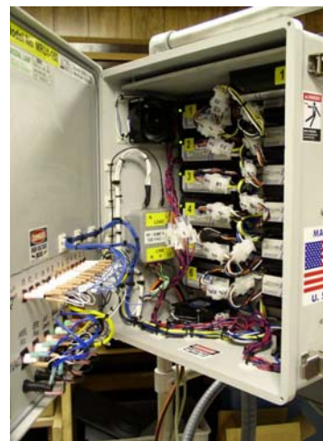
Figure 4. Photo of the Electrical Cabinet for the Pilot Unit
