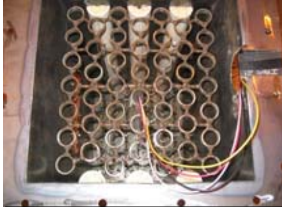
Photo No. 23. Top Support Rack – Showing One UV Bulb Assembly with its Connecting Wires
