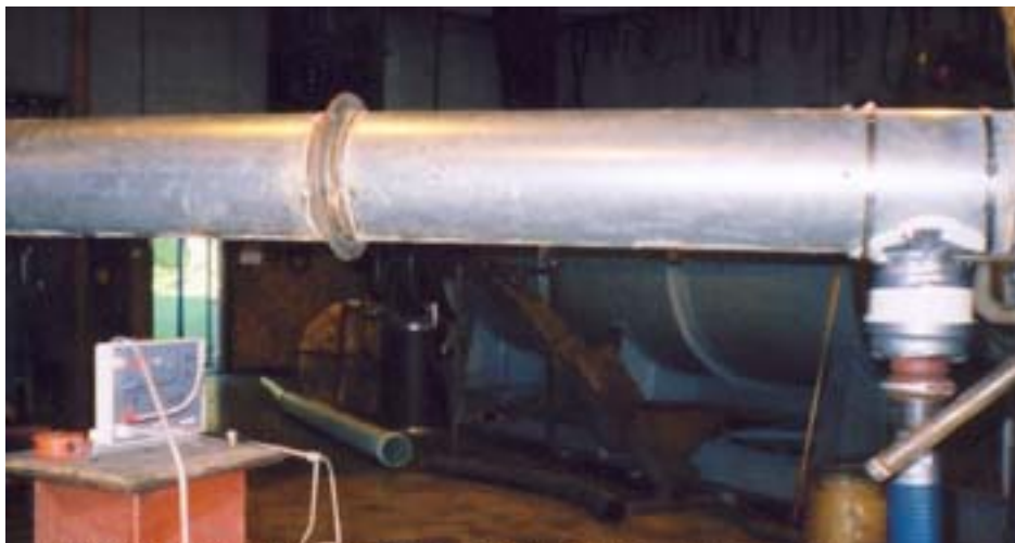
Photo No. 6. Fluidizing Airflow Monitoring Station
