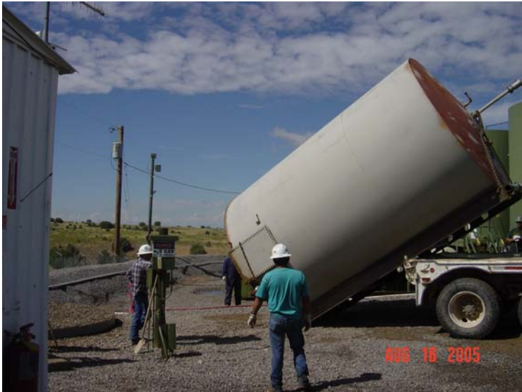
a) Placement of produced water tank outside of test building.
