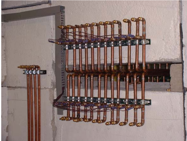
Figure 3-7 Cooling supply lines.
