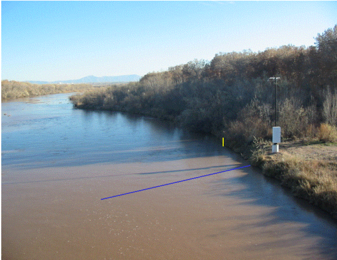
Figure 4.1: View of the Rio Grande TDR station from the Central Avenue Bridge. The Rio Grande TDR station consists of the Data acquisition/PV equipment enclosure mounted to a pole holding the PV panel. The pole is mounted on a 18-inch diameter concrete foundation. The approximate location of TDR probe #1 is indicated by the yellow vertical line downstream and against the right bank while the approximate location of the other 7 probes are indicated by the blue line extending out from the bank.
