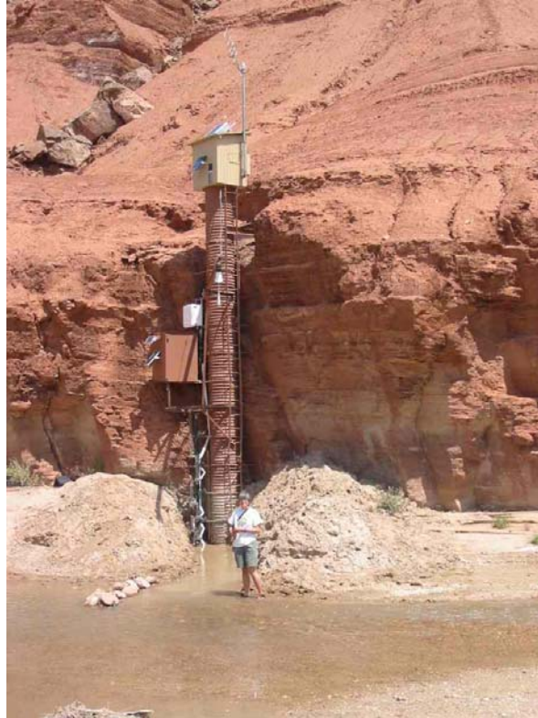
Figure 5.1: View of the USGS gauging station at the Paria. The TDR monitoring system is mounted on the frame work of the USGS station and consists of the white enclosure seen midway up the stilling station above the larger brown enclosure and a stack of TDR probes immediately to the left of the stilling station. See Figure 4.2 for a close-up view of the TDR stack.
