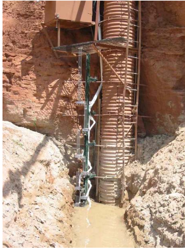
Figure 5.2: Close-up view of the TDR probe stack. Seven probes are visible with the top of the waveguides of the eighth probe barely visible at the water surface.
