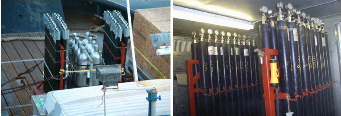
Figure 10.7.1 Pressure Vessels for Long Term Storage
