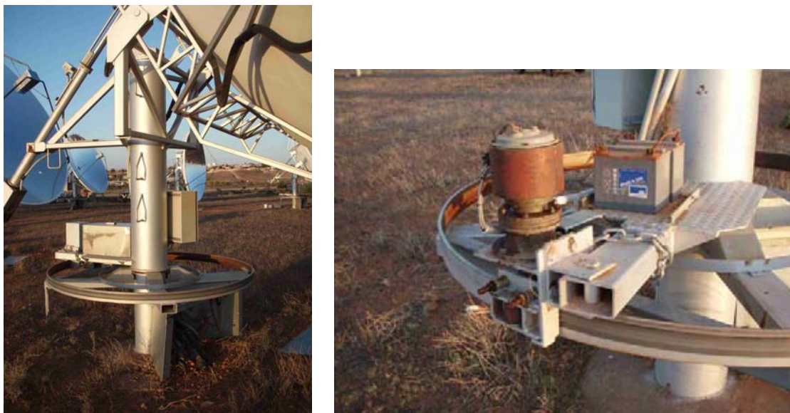
Figure 6-3. The “pipe-in-pipe” azimuth drives at White Cliffs required little maintenance during the 17-year operating history of the plant.
