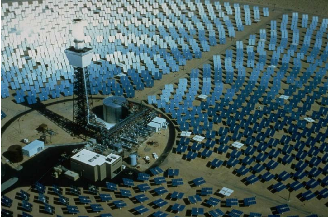
Figure 2-2. From 1982 to 1988, Solar One (near Barstow, California) used 1,818 pedestal-mounted heliostats built by Martin Marietta. Each heliostat was 39.1 m 2 for a total area of 71,130 m 2 . The heliostat field was used again during the Solar Two project from 1996 to 1999.
