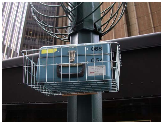
Figure 4. BATS Installed on a Light Pole.
