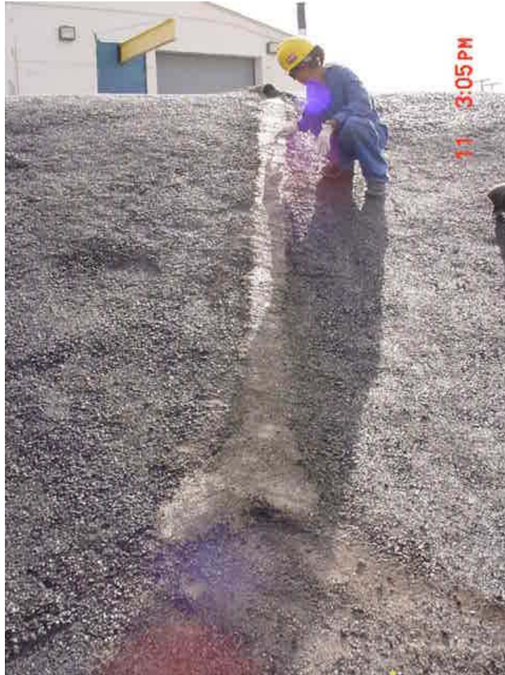
Figure B-3. Lower part of drain line over Site CPP-79 removed and depression filled in with concrete.
