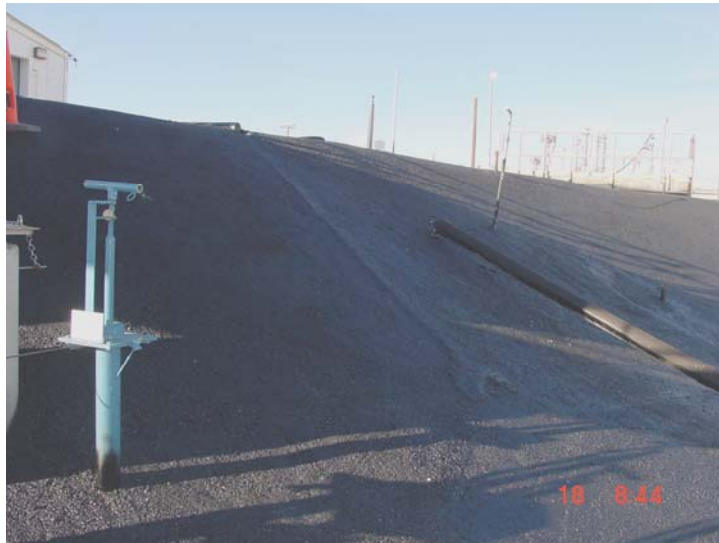
Figure B-4. Showing drain line over Site CPP-79 removed, depression filled in with concrete, and area sealed with seal coat.
