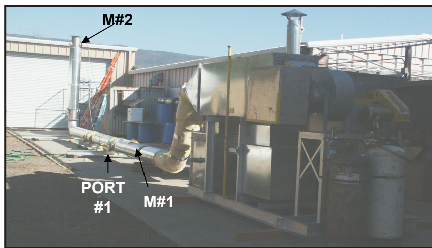
Figure 6. Variable temperature and flow system under test at STL
