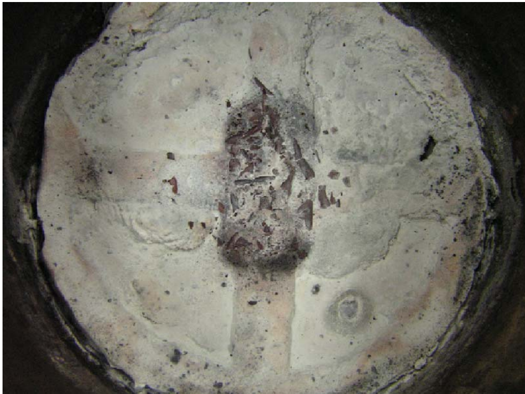
Figure 4.13 The solidified slag surface is not flat
