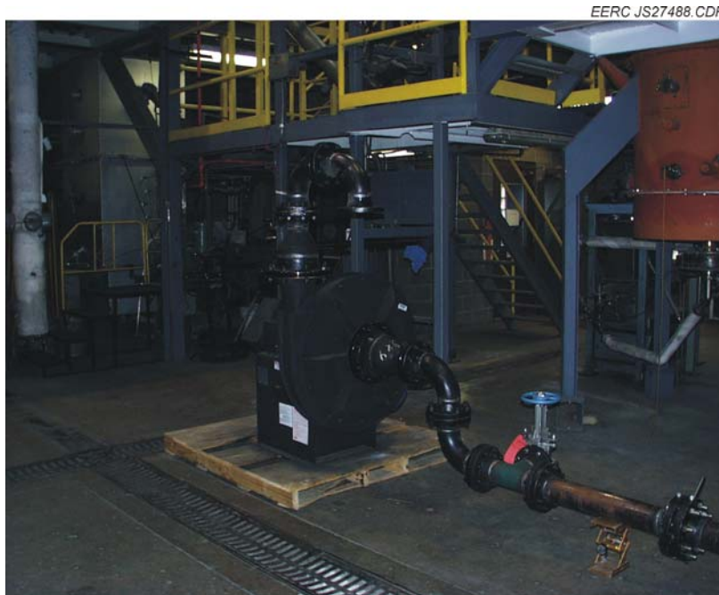
Figure 7. ID fan and TA control valve.
