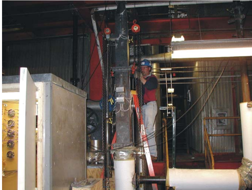
Figure 12. Installation of reactor chamber at test site with control room, reactor chamber, and piping visible.
