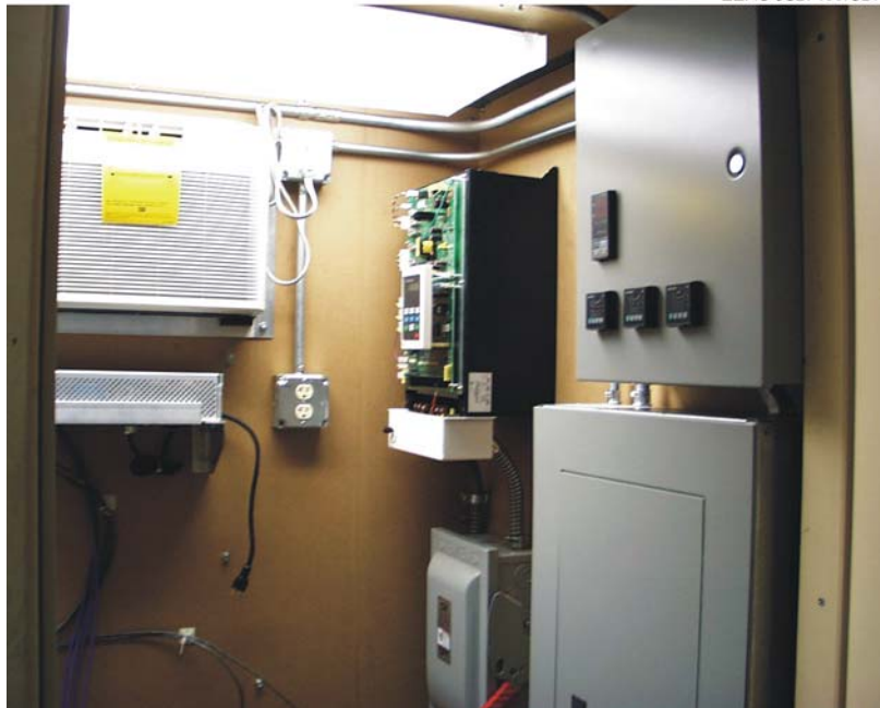
Figure 4. Interior SCR control room with air conditioner, several control boards, and breaker panel visible.
