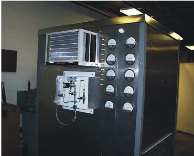
Figure 3. Exterior SCR control room with air conditioner, ammonia injection system, and manual pressure readouts visible.
