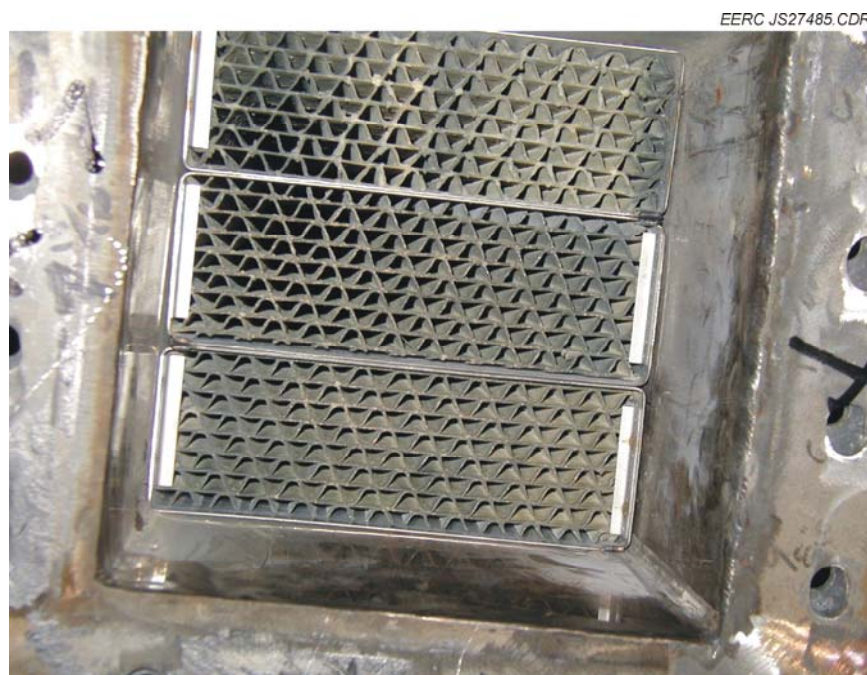
Figure 11. Clean, new SCR catalyst sections inside reactor chamber.
