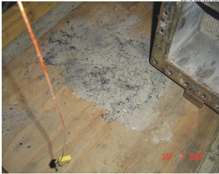
Figure 24. Ash containing black particles from top of SCR catalyst chamber.
