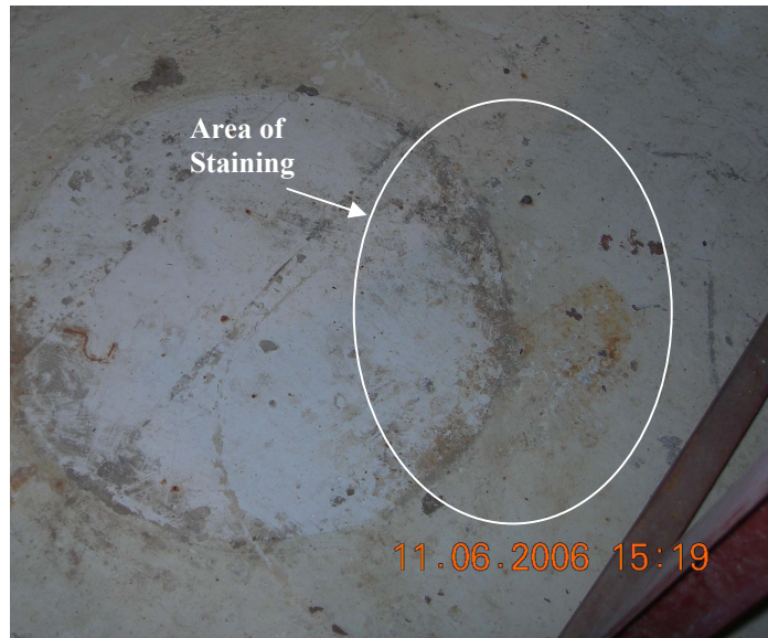
Figure 5. Photograph showing stained area associated with waste released from the failed pump gasket. Photograph was taken after receiver tank (99TRA00004) was removed.
