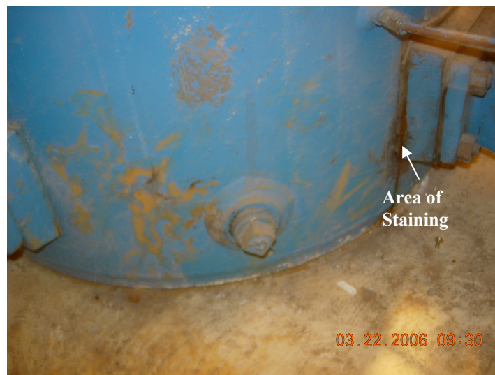
Figure 4. Photograph of the receiver tank (99TRA00004) and associated pump. The arrow identifies the release from the pump gasket.
