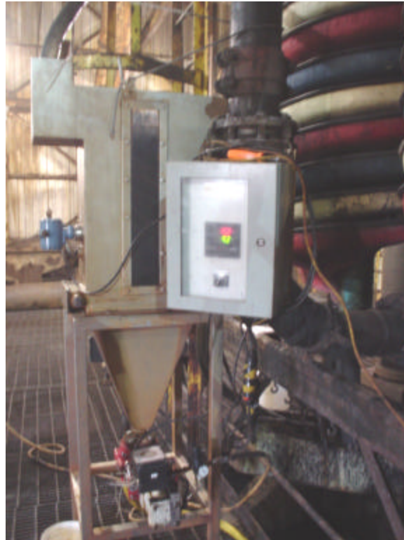
Figure 1.14. The 9x16-inch Pilot-Scale CrossFlow Test Circuit at Plant D.
