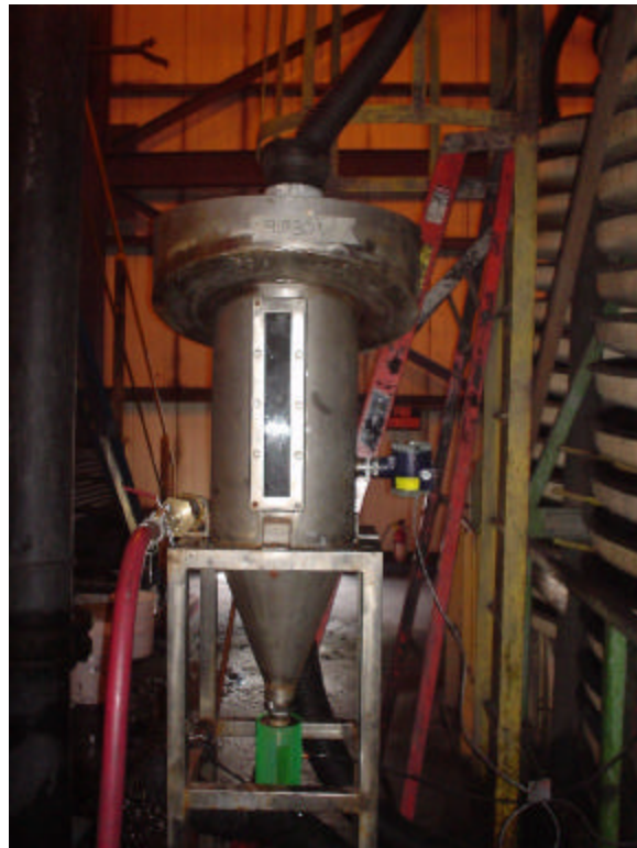
Figure 1.12. The 12-inch Diameter Pilot-Scale CrossFlow Separator Test Circuit at Plant C.
