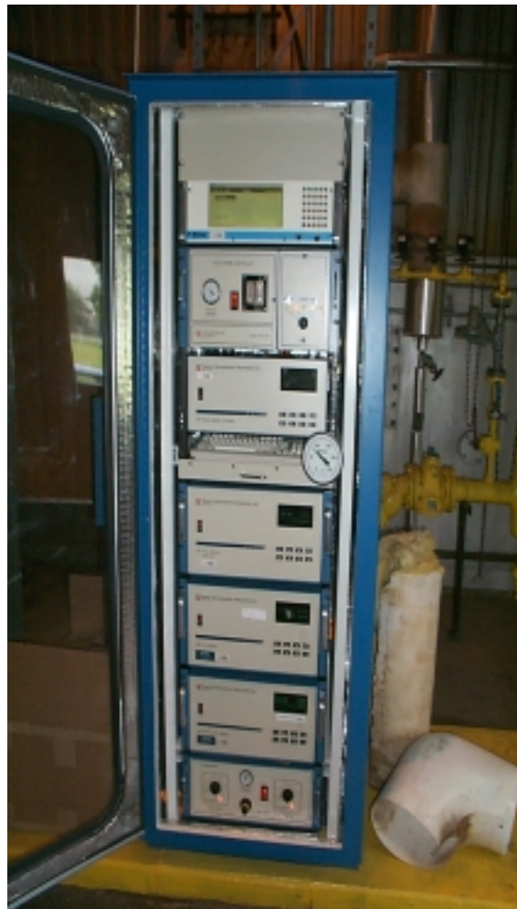
Figure 4-6. Central Steam Facility Continuous Emission Monitoring Analyzers.
