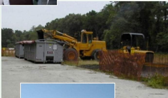
▶ Figure 2-13. Soil Removal. In October 1999, a layer of soil approximately six inches deep containing PCBs was removed from the Building 96 area.
