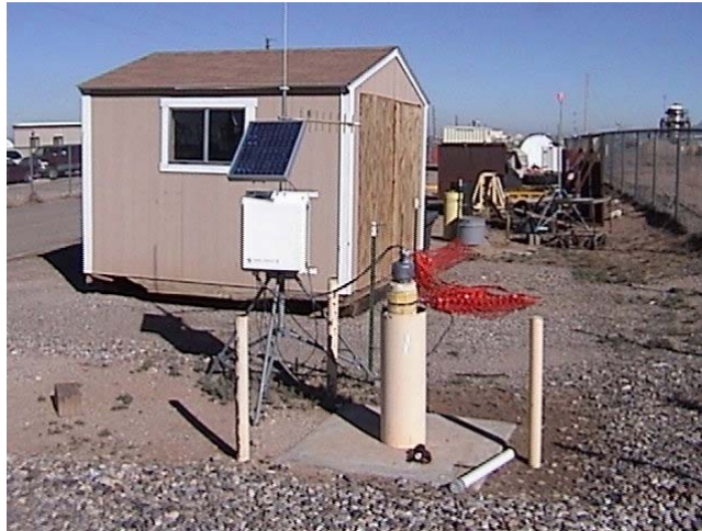
Figure 71. Solar-powered remote data-logging stations next to well D3 at the Chemical Waste Landfill.
