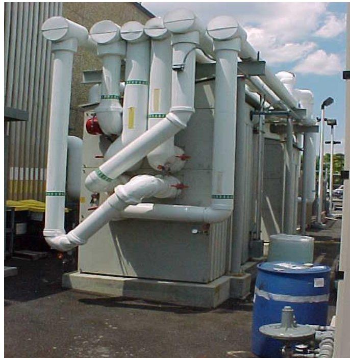
Hot Water Absorption unit
