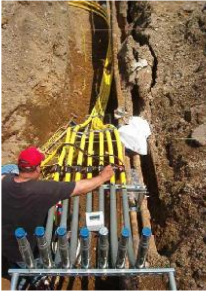
Natural gas distribution lines to fuel cells
