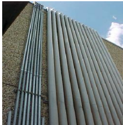
Piping and structural supports for air cooled condensers and electrical conduits
