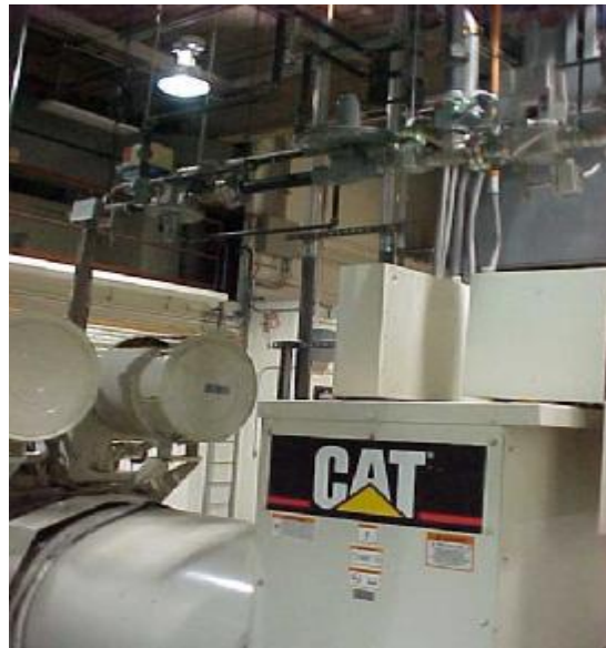
Natural gas train on bi-fueled diesel engine
