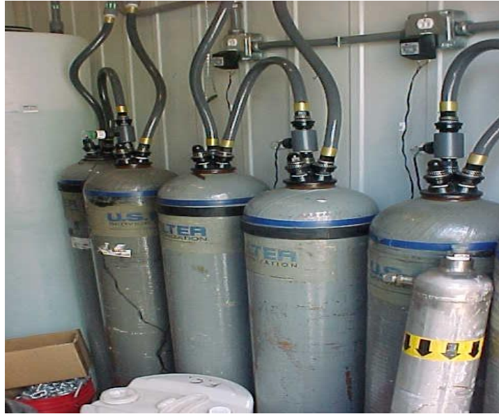
de-ionizing system to fuel cells
