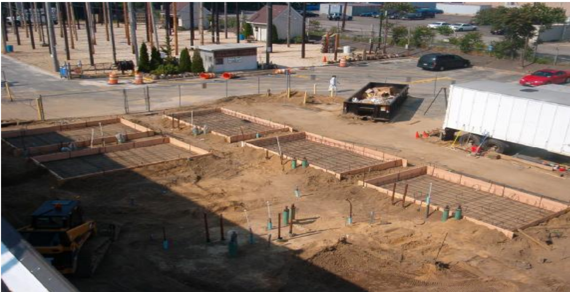
Piping to and from fuel cells and foundation forms for the fuel cell modules
