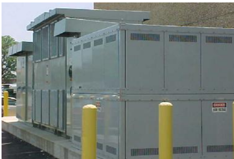
High Voltage entrance – 13,800V Isolation transformer and neutral grounding reactor
