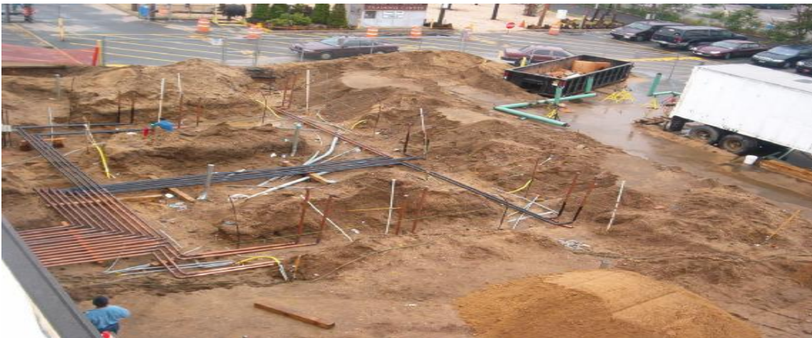
Piping installed at various elevations
