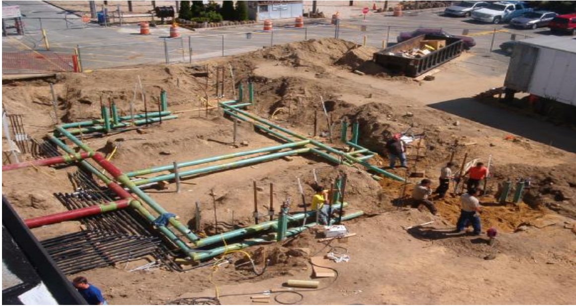
HGHW lines overlaying subterranean piping
