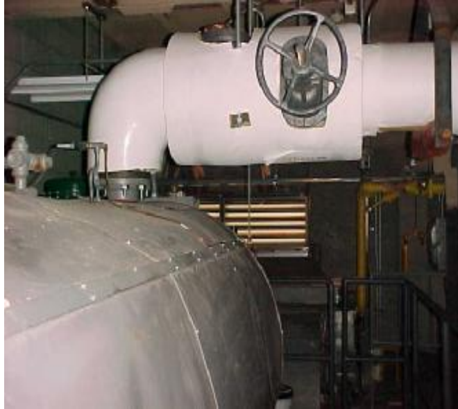
Steam Generator in boiler room
