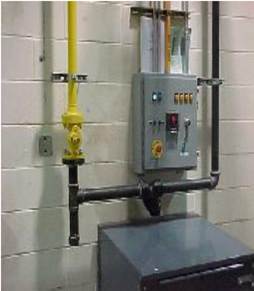
Natural Gas service entrance into diesel room
