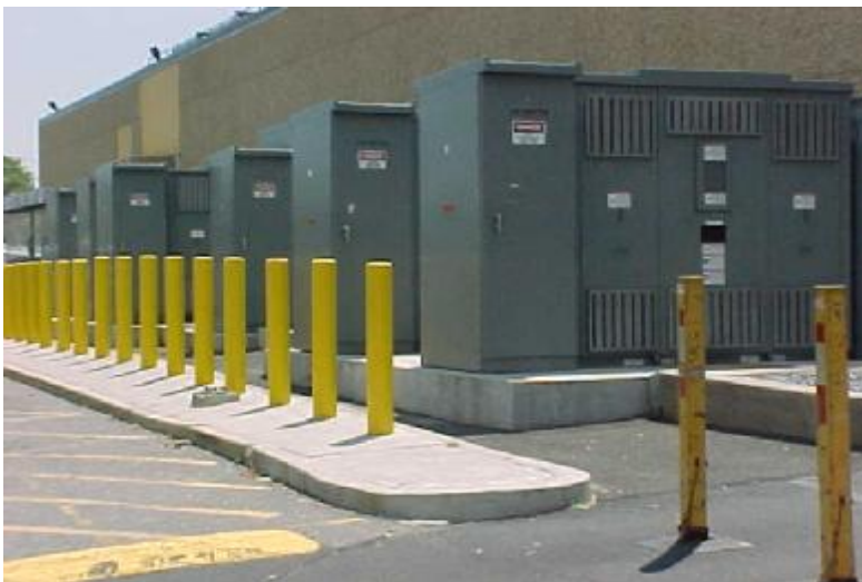
Transformer bank in parking lot
