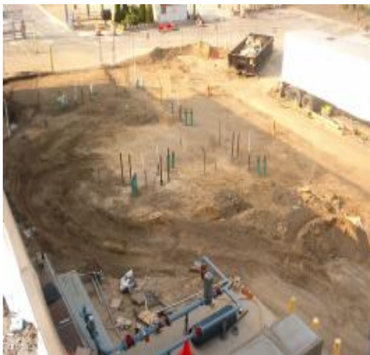
Subterranean piping extending up to fuel cell foundations
