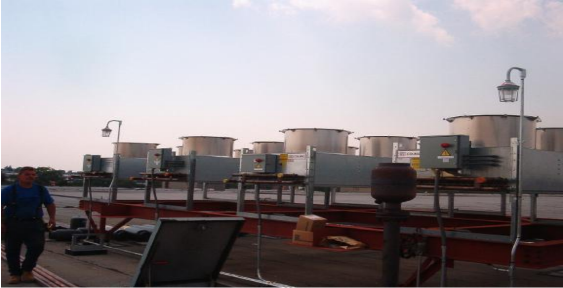
Roof mounted Air Cooled Condensers
