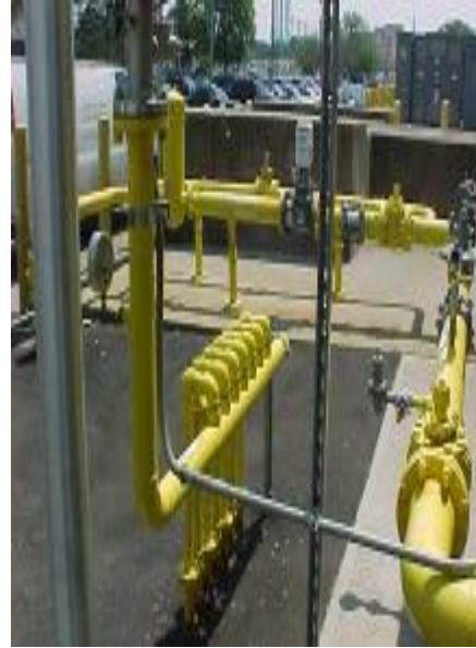
Natural gas meter and manifold to fuel cells
