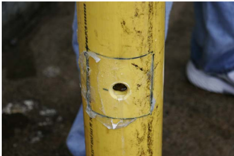
Figure 25: Failure of adhesive patch during quick burst testing at 450 psi
