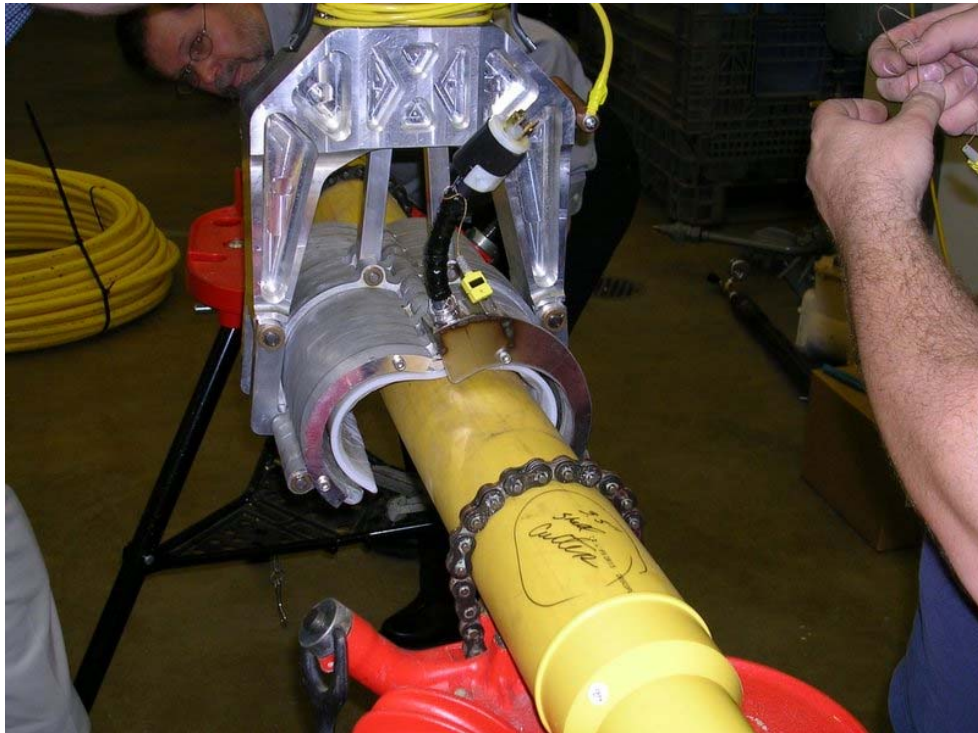
Figure 49: Engineered prototype with PE gel film repair patch being applied to damaged 4-inch MDPE pipe
