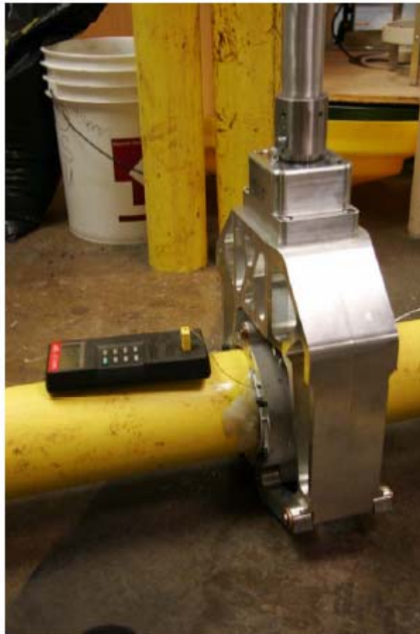
Figure 28: Overlapping full-wrap patch applied to 4-inch MDPE pipe during demonstration for Northwest Natural
