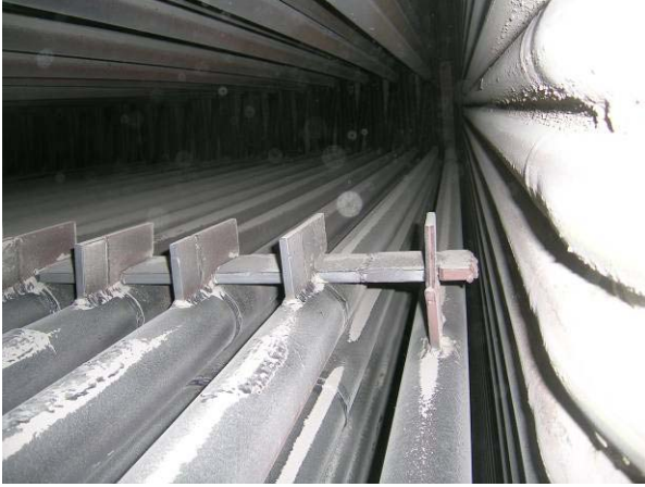
Figure 6. Secondary superheater tubes and supporting brackets. In this picture, the view is looking up words along the superheater tubes (lower left). The tubes on the right are part of the membrane wall.
