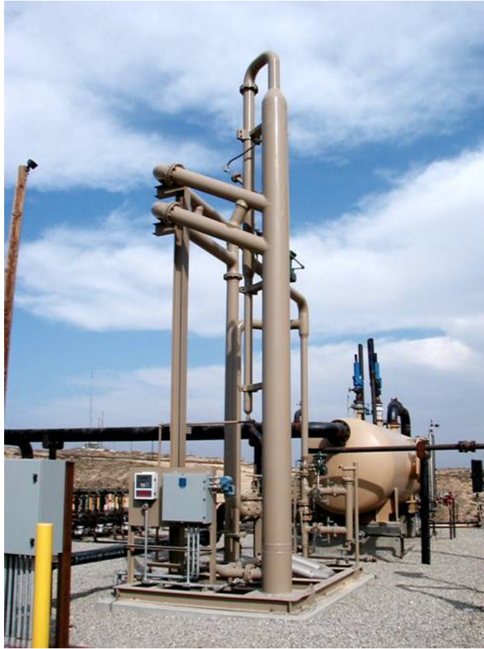
Figure 26 – GLCC ® -Slug Damper (SD) System Installed in California (Courtesy: System Measurements Services)
