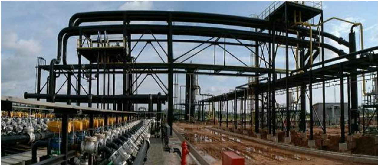
Figure 25 – Dual GLCC ® -Slug Damper (SD) System Installed in the Field in Indonesia (Courtesy: Chevron)
