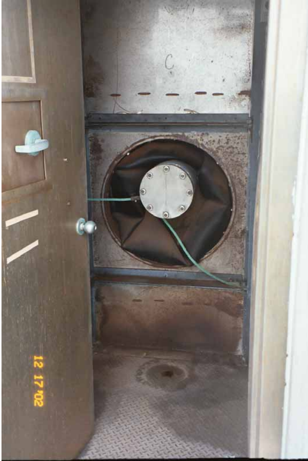
Figure 7. Stack sampling port
