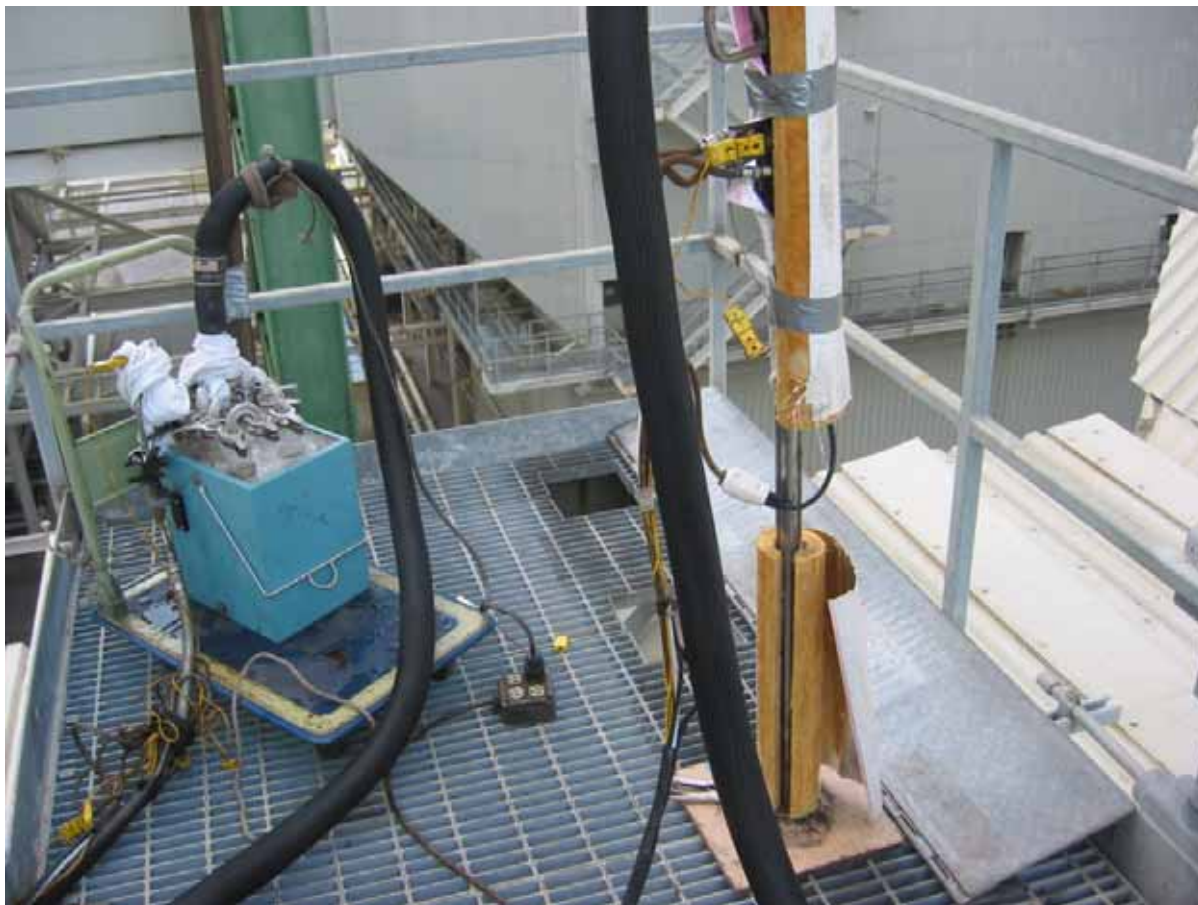
Figure 5. ESP inlet (air heater outlet) probe and sampling train
