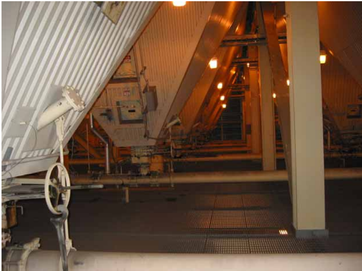
Figure 9. ESP ash hoppers, showing pipes used for transferring ash to the silo
