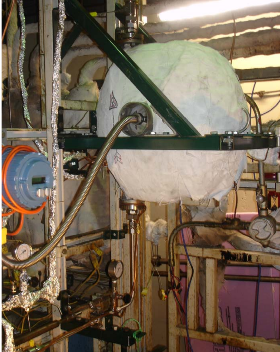
Figure 4. The Newly Installed Slurry Flowmeter.
