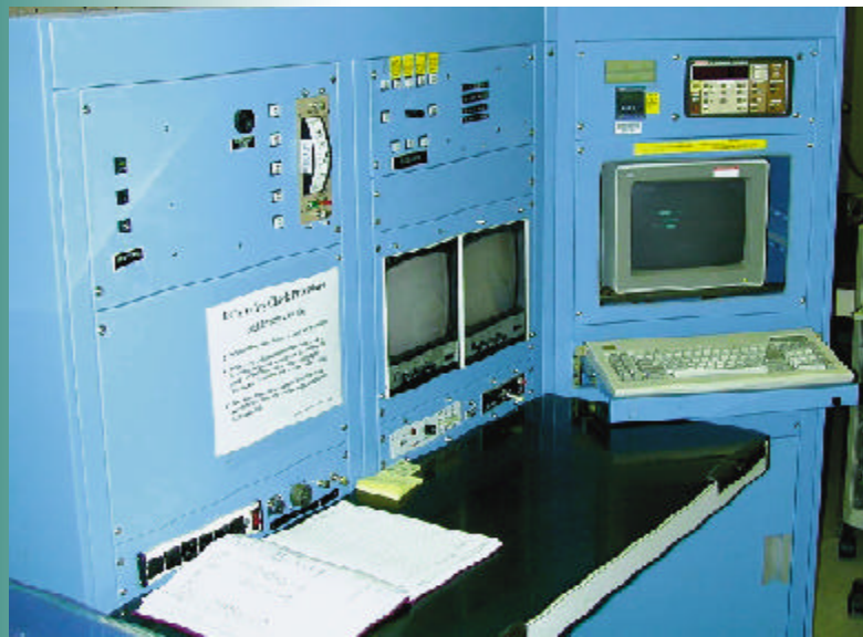
Figure 2.15. The High-Exposure Facility Control Room. The facility remotely controlled from the panel shown above, which also houses the monitors for remote cameras within the radiation area and allows for remote positioning of instruments, once the 1-m offset is established using the positioning lasers.
