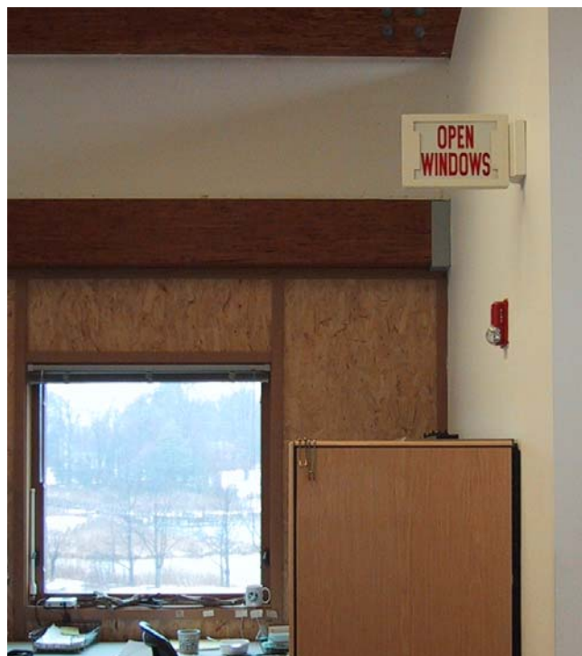
Figure 3-26 Signage at CBF directs occupants to operate windows
