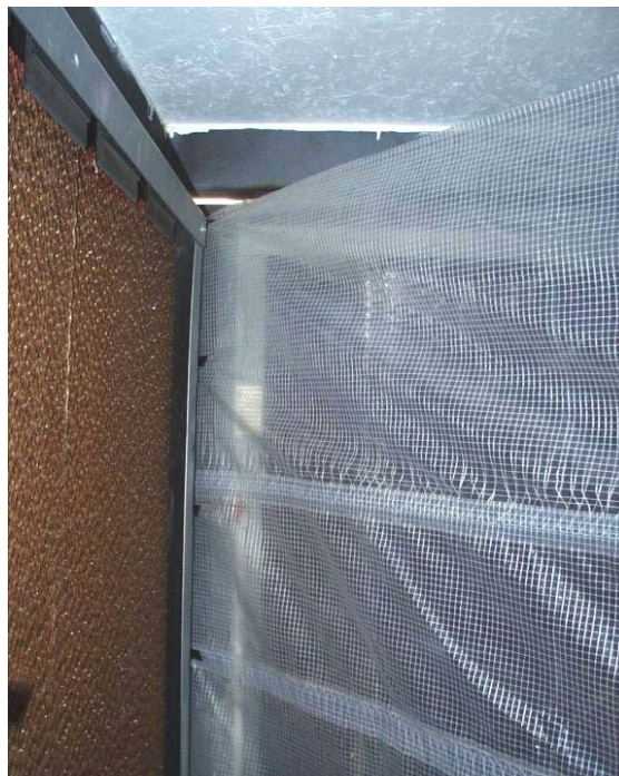
Figure 3-31 Plastic blocking device for cooltowers
