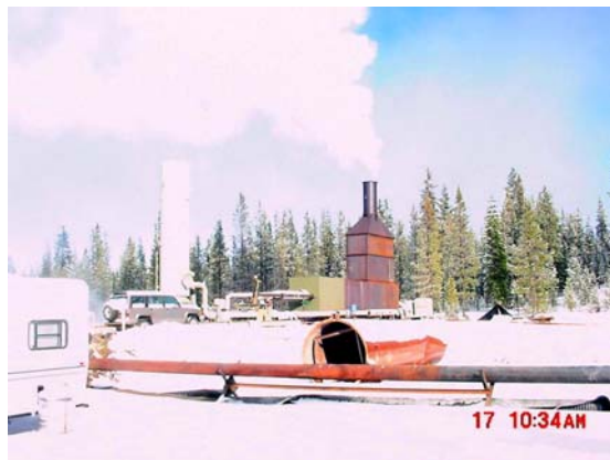
LEAMS III Separator at California Geothermal Field
