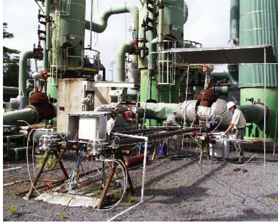
Figure 3. Apparatus installed at Puna for testing coated tubes exposed to injection fluids.
