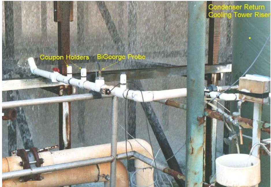
Figure 2. BIoGEORGE™ Biofilm Activity Monitor installed at the Aidlin cooling tower.
