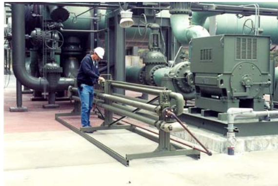
Figure 2. One of two sidestream skids used at Mammoth for testing coatings exposed to production and injection fluids.
