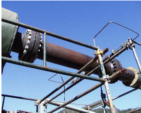
Figure 4. PPS-coated caustic injection spool installed at the Aidlin plant at the Geysers.
