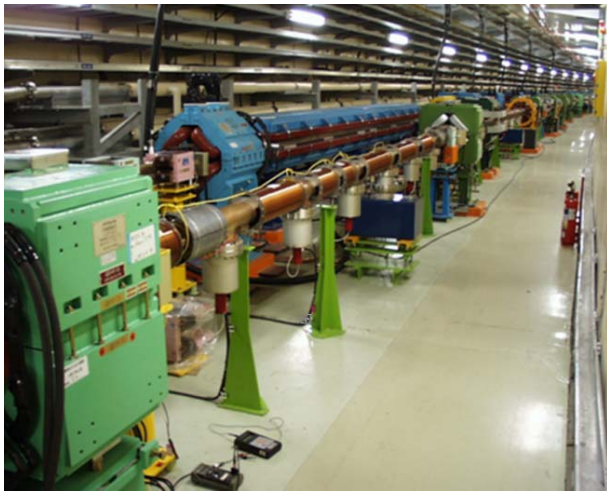
Figure 4 Tunnel view of KEKB
