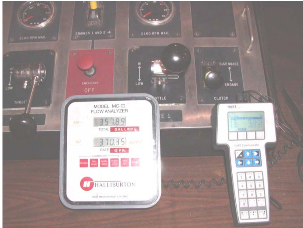
Figure 7 Flow Control Console, Flow Meter and Pressure Readout
