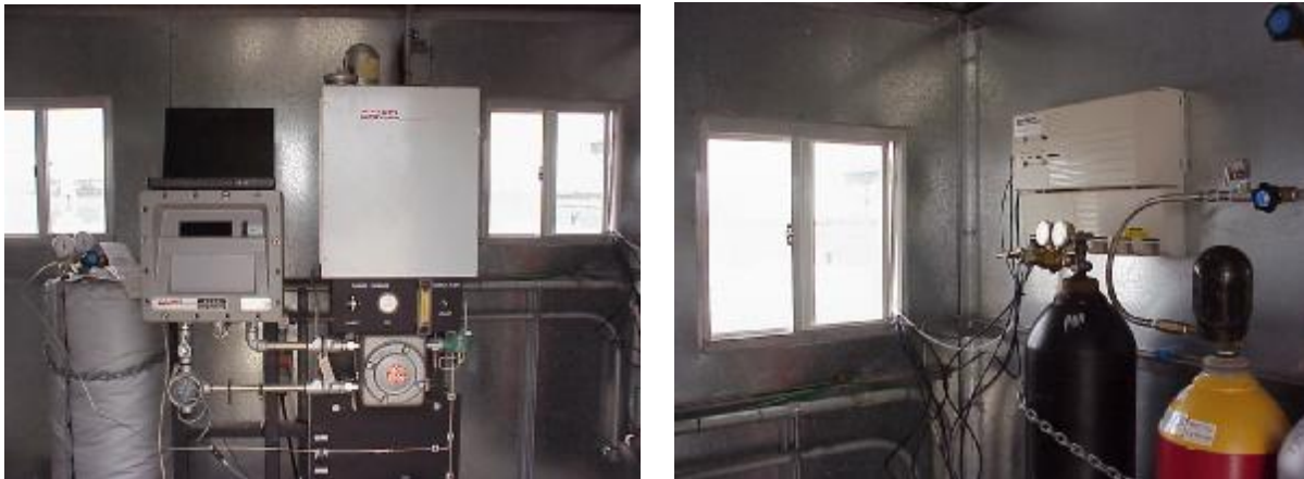
Figure 6-26. Field site enclosure for the on-site gas chromatograph (left) and the energy meter Bristol Babcock flow computer (right).
