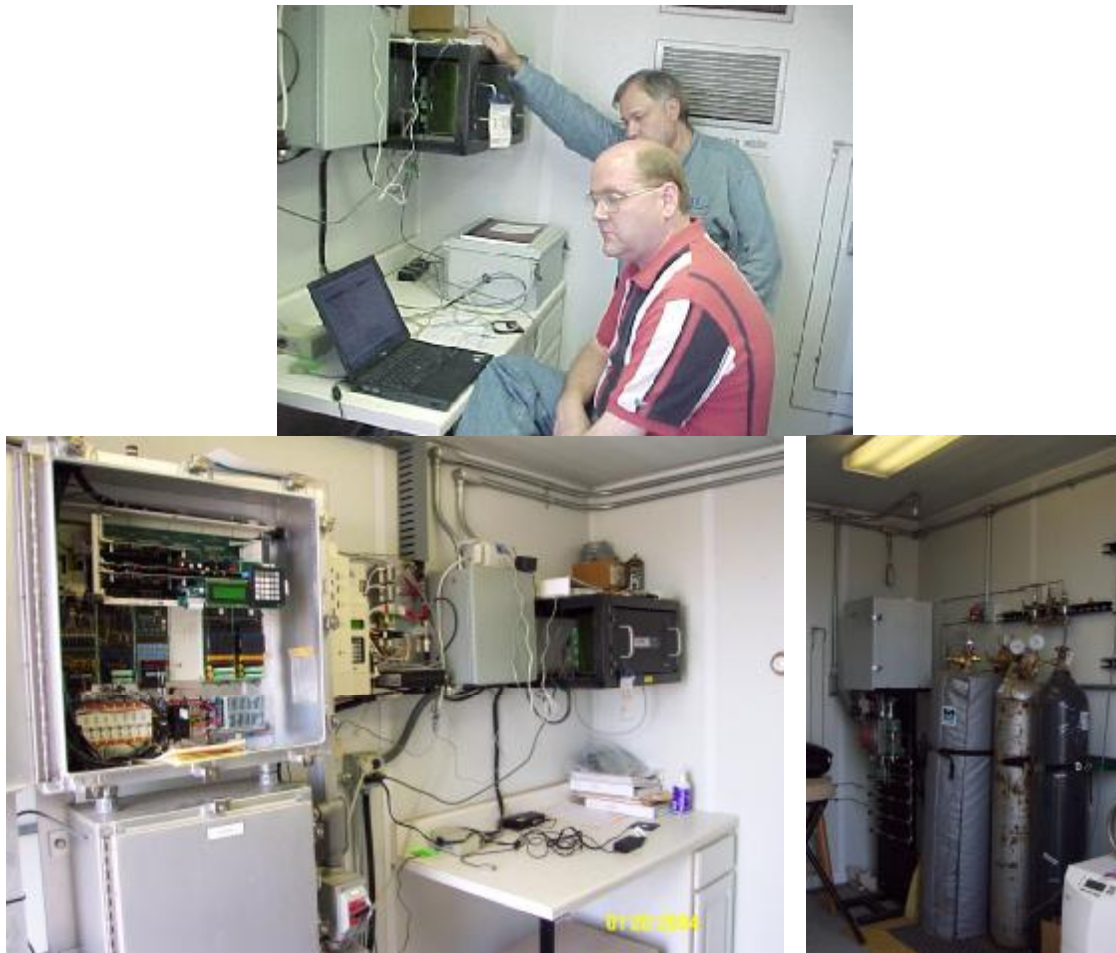
Figure 6-33. Installation of the RGC data logger at the El Paso field site. Top : RGC data logger (on the workbench) implementing the algorithm. Bottom left : Flow computer and data connections providing sound speed, temperature, and pressure data. Bottom right : Chromatograph providing diluent data.
