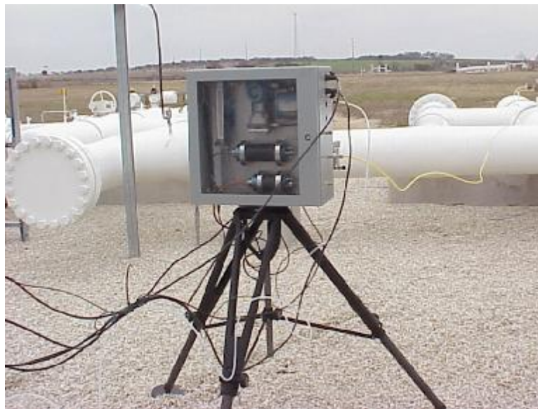
Figure 6-25. Front view of the energy meter module installed at the New Braunfels, Texas field site.
