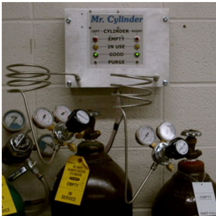
Figure 5: Mr. Cylinder system for automatically switching between argon gas bottles for the annealing oven.
