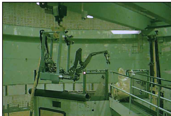
Fig. 9. DAWP working above the CP-5 research reactor.
