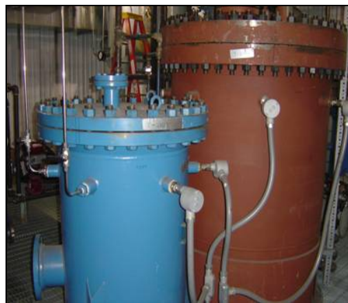
Figure 16 – Stage II Fine Sorbent Feeding System Pressure Vessels
