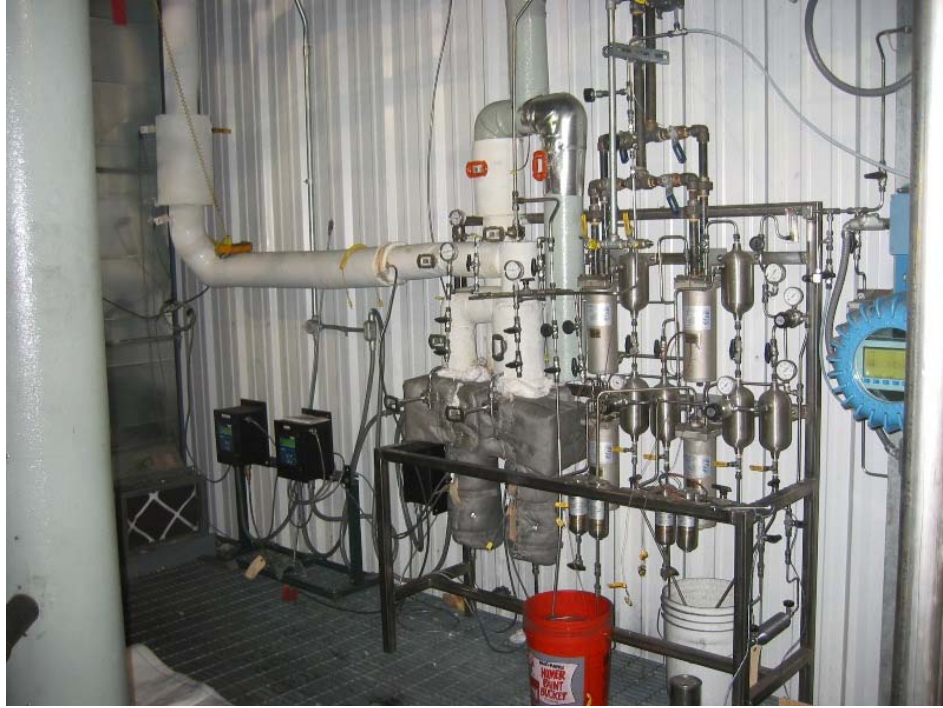
Figure 18 - Main FFTF Sample Extraction and Conditioning Skid (Untreated Syngas)
