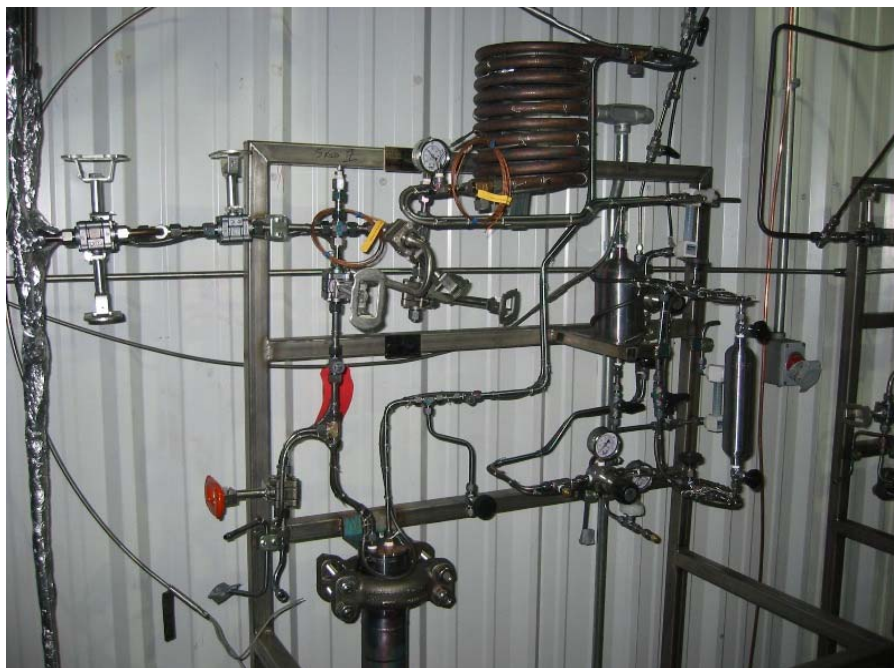
Figure 21 - Photograph of the SE&C Skid #2 at the G-13/G-14 Locations (Before Insulation)
