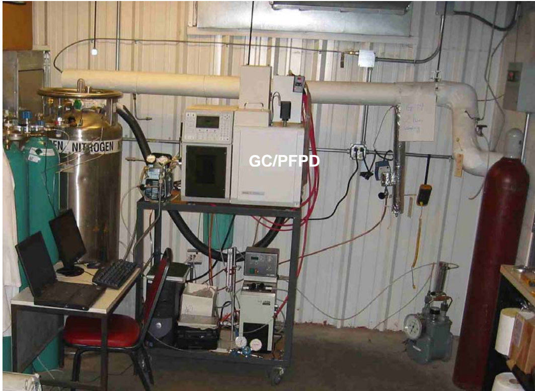
Figure 27 – Flex-Fuel Test Facility Fourth Floor Analytical Station
