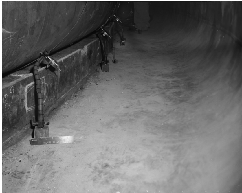
Fig. 4. Strain gage monitoring in tank SY-103 to assess impacts from primary bottom bulges.
