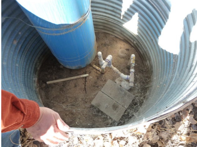
Figure 8. The currently unused water supply well to the northeast of the north lake.
