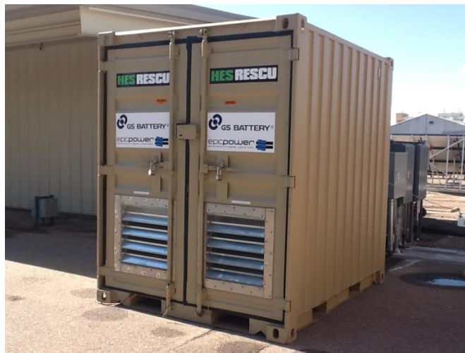
Figure 1 GS Battery, EPC Power energy storage system delivered to Sandia
