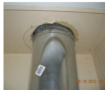
Fig. 6. Gap around flue as it enters attic should be sealed with sheet metal on the floor of the attic. Follow all fire code requirements—these vary depending on type of flue (single, double, insulated, etc.).
