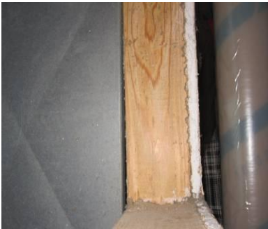
Fig. 76. Crack in return plenum (between metal and wood).
