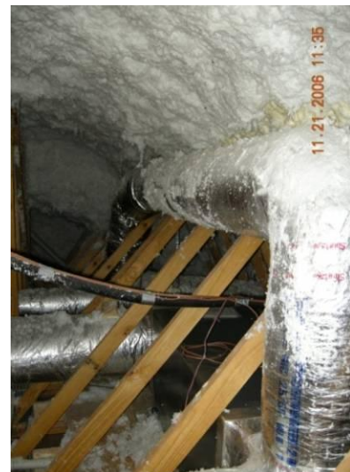
Fig. 27. Air conditioning unit inside attic insulated with spray foam and spray fiberglass.
