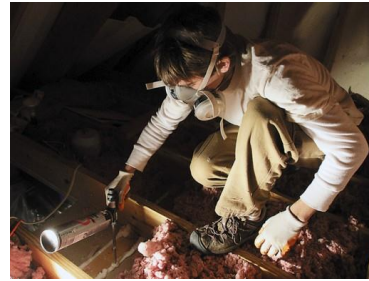
Fig. 4. Contractor seals an interior wall top plate in the attic. Photo: Chad Greene.
