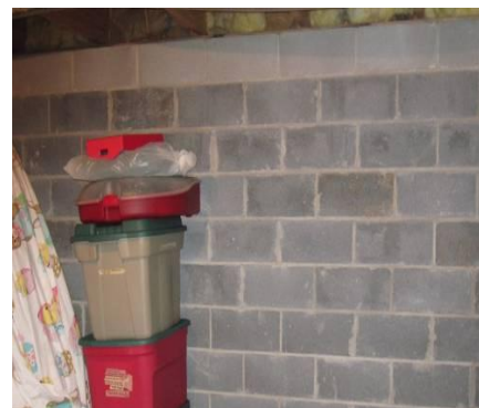
Fig. 41. Uninsulated cinder block basement and band joist.
