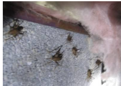
Fig. 78. Uninsulated ductwork in crawlspace with crickets feeding on mold growth.
