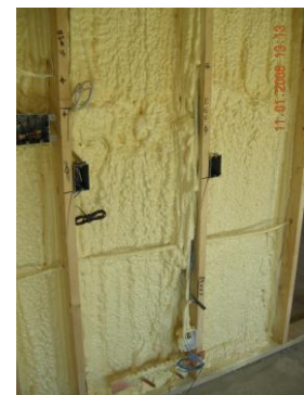
Fig. 11. Wall between the garage and kitchen in energy-efficient house. (Flash-and-batt walls form good air seal between garage and kitchen.)
