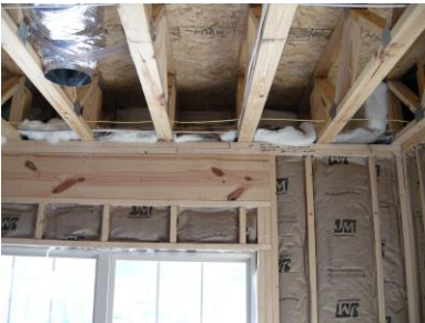
Fig. 12. Cantilevered floor improperly insulated and sealed.
