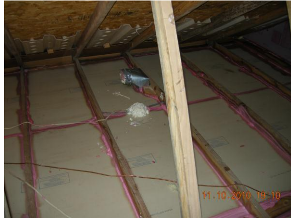
Fig. 43. Sealed and reinsulated attic. (The fiberglass batts were removed and used in the crawl space under the office. The attic was vacuumed, the electric outlets were foamed with GREAT STUFF™, and the remaining cracks sealed with the pink EnergyComplete™ latex foam.) Then new insulation was blown in to create an R-value of 60.
