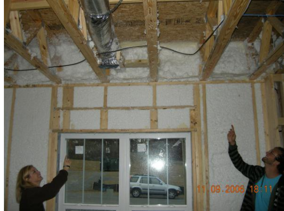
Fig. 21. Flash-and-fill done correctly in cantilevered floor. (Note the closed-cell foam under the second floor right above the blown in fiberglass.)
