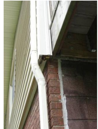
Fig. 60. Rim joist/sill area needs to be sealed and insulated.
