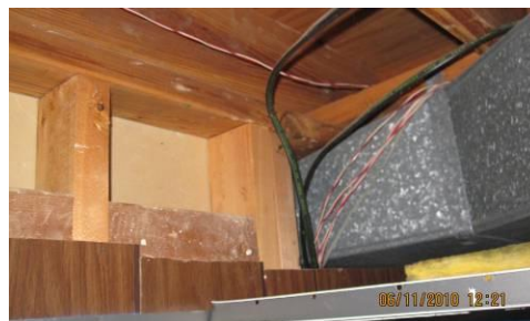
Fig. 34. Open wall cavities, ductwork, and electrical penetrations support unwanted air flow.
