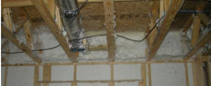
Fig. 14. Flash-and-fiberglass insulation under cantilevered floor system provides air-tight construction in high-energy-efficiency house.
