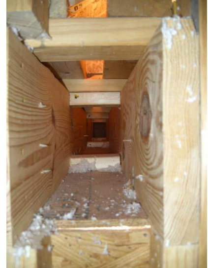
Fig. 30. Box beam penetrating house.
