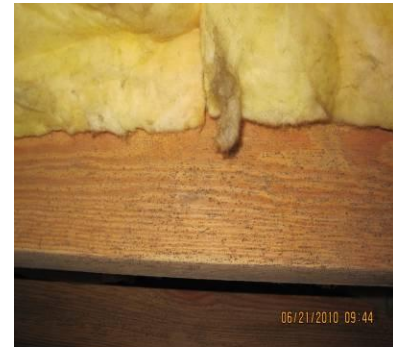
Fig. 73. Moisture allows mold to discolor the floor joist.
