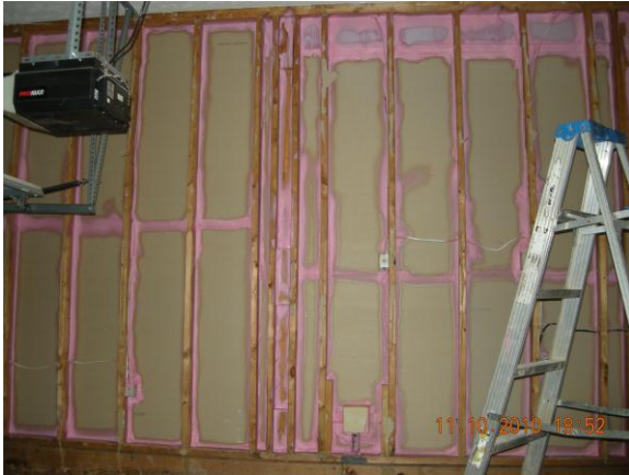
Fig. 42. Owens Corning EnergyComplete™ is used to improve the air barrier between the garage and the conditioned space.
