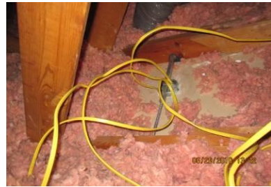
Fig. 79. Patchy, loose insulation in the attic.
