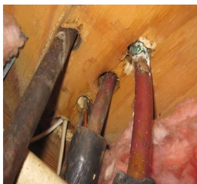
Fig. 68. Electrical and plumbing penetration provide airways between the house and the crawl space.
