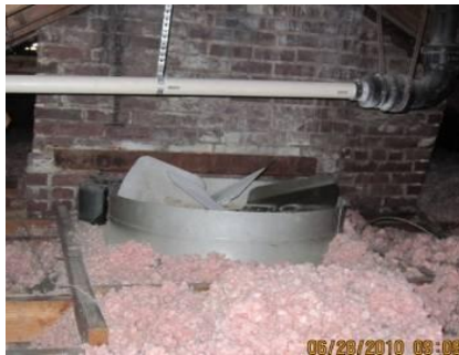
Fig. 65. Fan and gaps around chimney allow air to move freely between house and attic.
