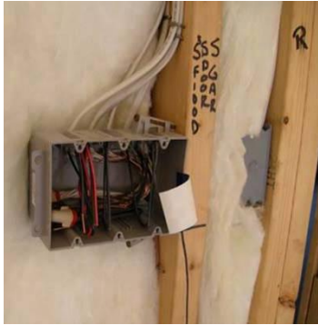
Fig. 28. Electrical box compressing insulation and lacking seal.
