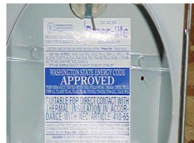
Fig. 20. Label showing electrical fixture is “approved for direct contact with thermal insulation.”
