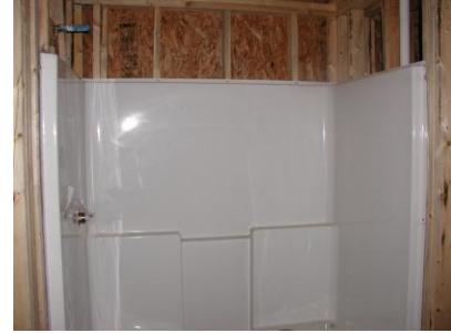
Fig. 9. No backing behind shower.
