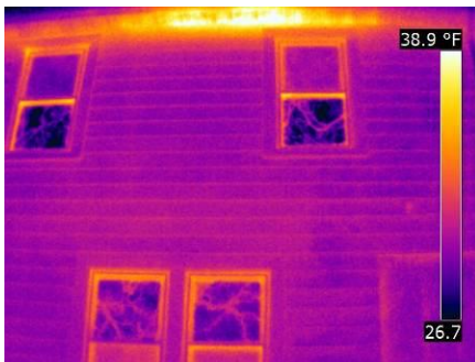
Fig. 53. Bright area indicates less effective insulation and sealing of soffit vent.
