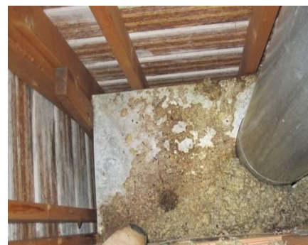
Fig. 40. Uninsulated chimney enclosure.
