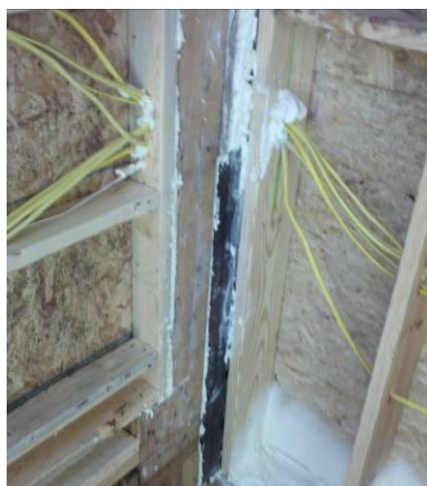
Fig. 37. Spray foam used to seal band joist, openings in framing, and electrical penetrations.
