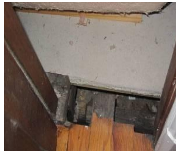
Fig. 66. Soiled flooring from air movement in wall.
