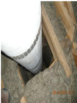
Fig. 71. Utility penetration into unconditioned attic.
