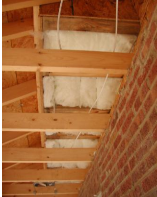
Fig. 13. Improperly insulated cantilevered floor from outside.
