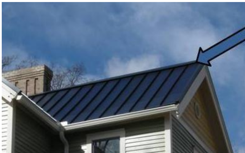
Photograph of 1.4 kW peak laminate PV designed to blend in with the standing seam metal roof.
