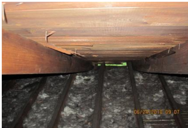
Sparse attic insulation before the retrofit
