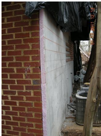
Above-grade basement walls shown during retrofit with foam board and the thin brick veneer being installed.
