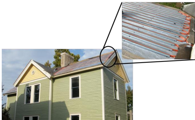
PEX tubing of the solar water heater collector installed underneath the metal roof.
