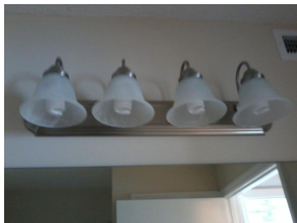
Fig. 18. New CFLs in a bathroom vanity fixture.
