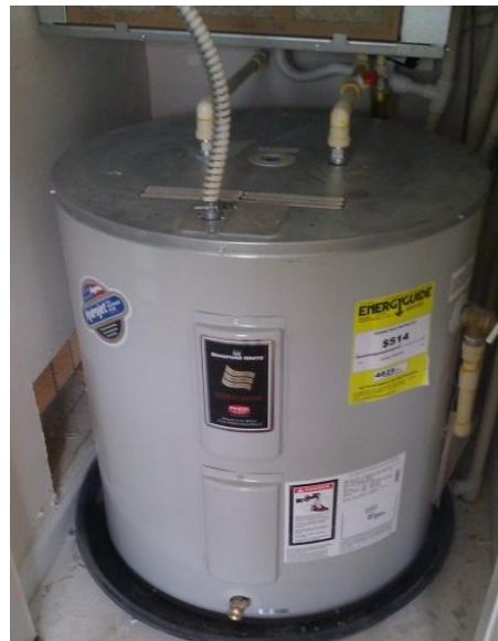
Fig. 14. New domestic water heater.
