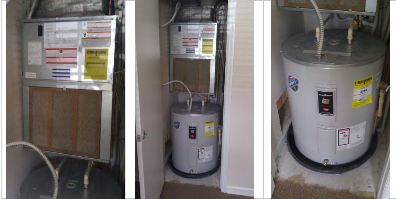
HVAC and DHW systems
