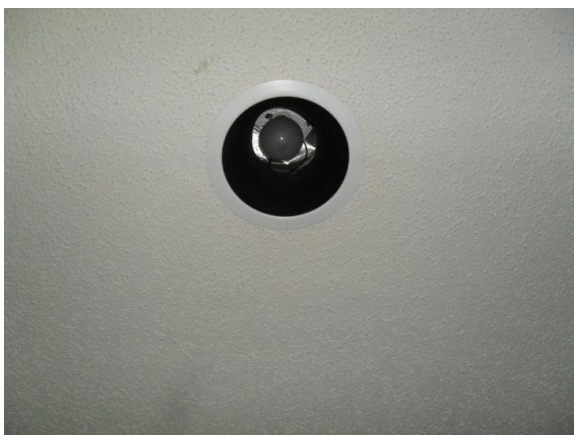
Fig. 17. Existing incandescent lamp in a recessed lighting fixture.
