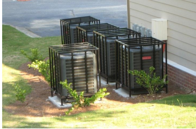
Fig. 12. New outdoor units of the heat pump.
