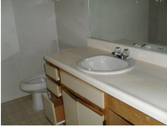
Fig. 15. Existing plumbing fixtures
