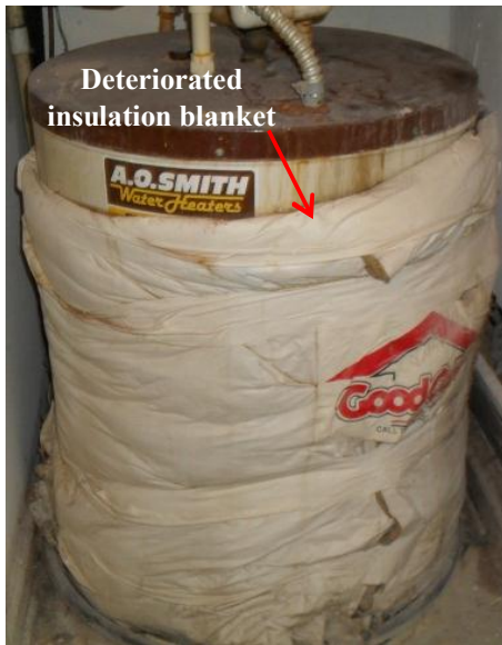
Fig. 13. Existing domestic water heater.
