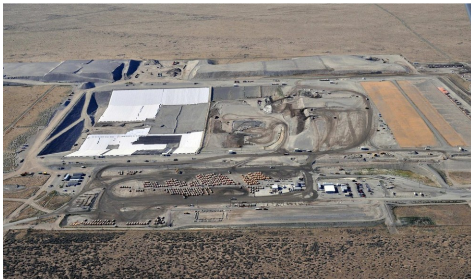
Fig. 1. Environmental Restoration Disposal Facility at Hanford during construction of liner and leachate system for new cells (DOE Photo).
